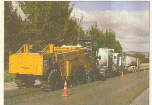
FULTON HOGAN'S recycling machine in action on State Highway 2 in the Hawkes Bay area of New Zealand.
